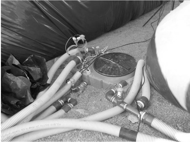
Figure 14: The well and pipes conveying in/out.
