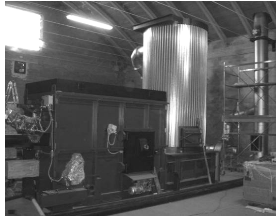
Figure 5: Picture of the diathermic oil boiler
