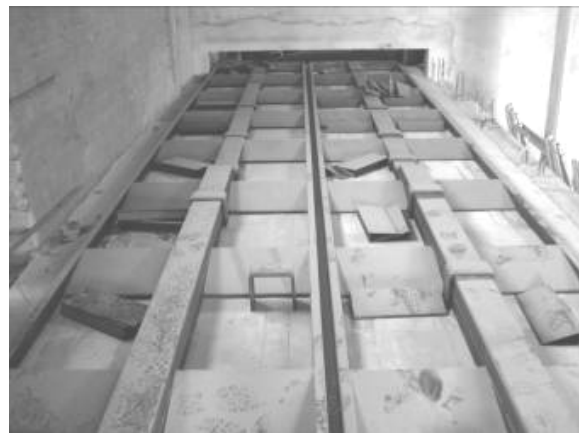
Figure 3: Moving racks anchored on the suspended floor
