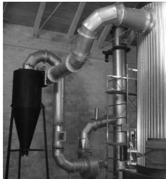
Figure 6: Picture of the exhausted gas cleaning and ejection system
